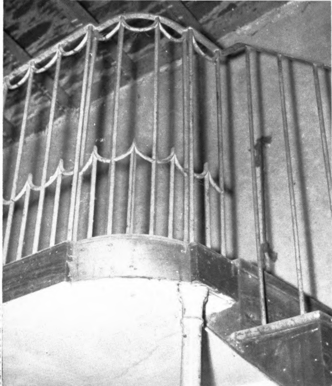
Page 126 (left) Detail of musicians' gallery in the School, showing refined workmanship characteristic of the building as a whole; (below) interior of No 3 mill showing the aisles of cast-iron columns and jack-arch construction. This photograph was taken during the clearing of the mills after closure in 1968
